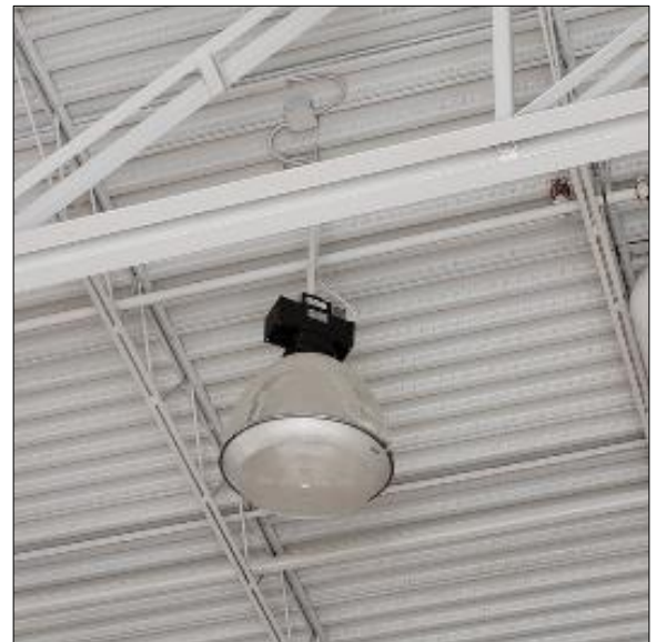
Photo E12: Typical Basketball Court Lighting Fixture
