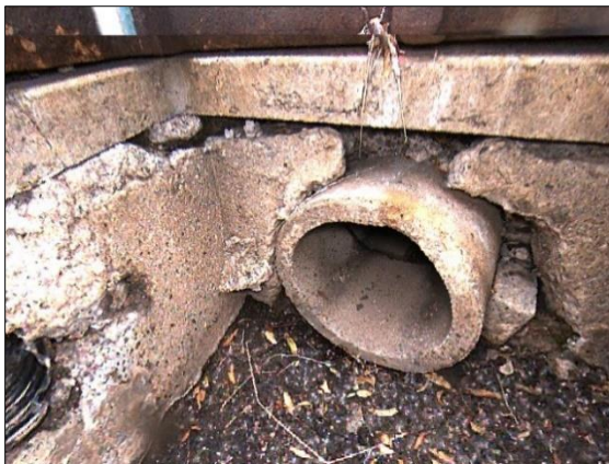
Photo C51: CB 6: Structure Damaged
