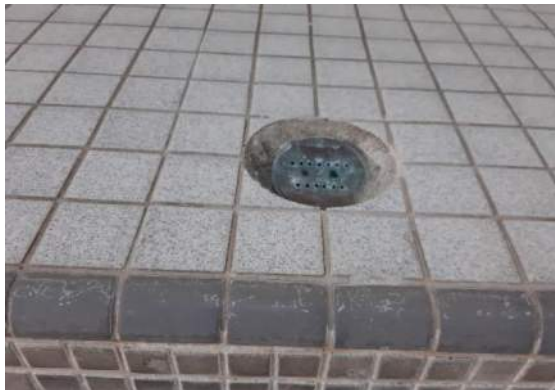
Figure 34 – Main Pool Spray Feature at Deck
