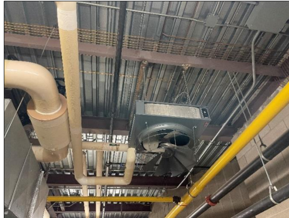
Photo M12: Typical Unit Heater
