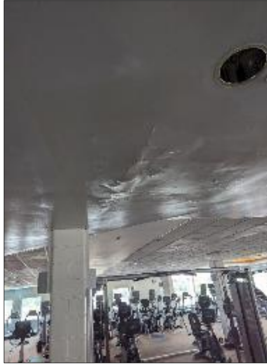
Photo ST 6: Signs of ceiling water damage.
