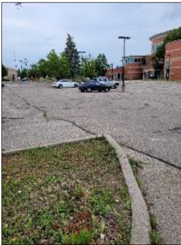
Photo C1: East parking lot closest to building looking south from north end. Longitudinal cracks, some sealed and grass growing in others. CB3 just east of light standard.
