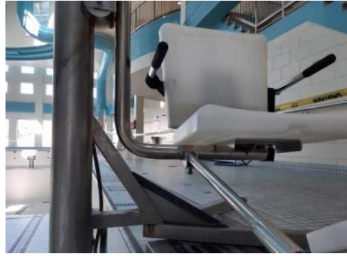
Figure 36 – Main Pool Accessibility Lift
