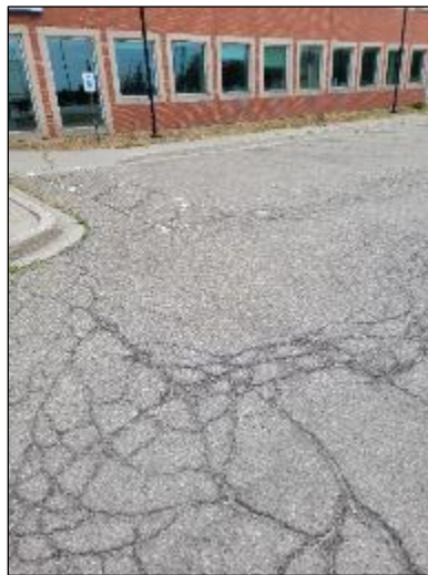
Photo C14: South Entrance – Alligator cracking, loss of asphalt.
