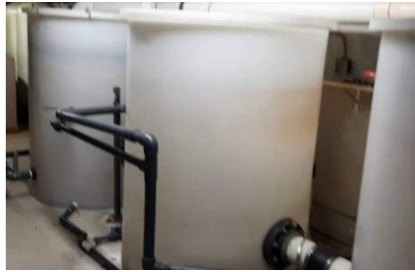
Figure 2 – Splash Pad Balance Tanks
