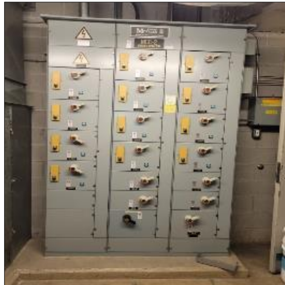
Photo E6: MCC 2 in Basement
