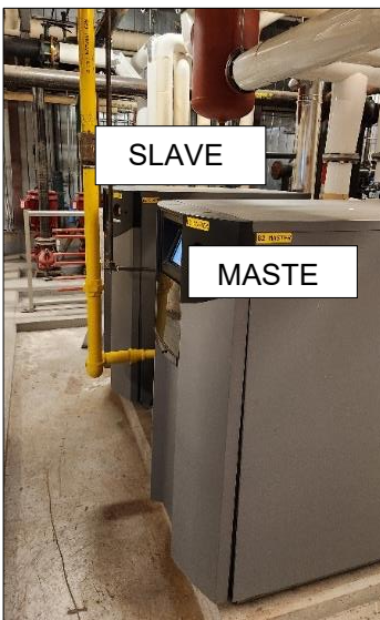
Photo M5: Boilers # 2 and #3
