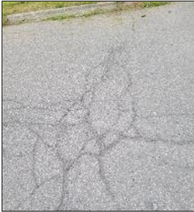
Photo C11: West Parking – Longitudinal and alligator cracks, loss of asphalt.
