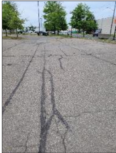
Photo C7: North Parking looking west from area of transformer. STMH 4 and CB6 in background. Longitudinal cracking, some previously sealed and sealing failing.
