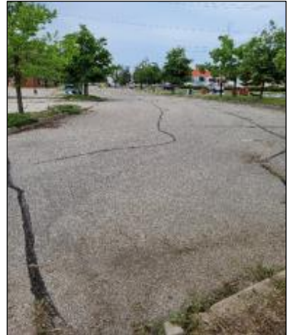
Photo C6: North Parking Lot looking west from northeast corner of the lot. Cracking, some previously sealed, grass growing in some.
