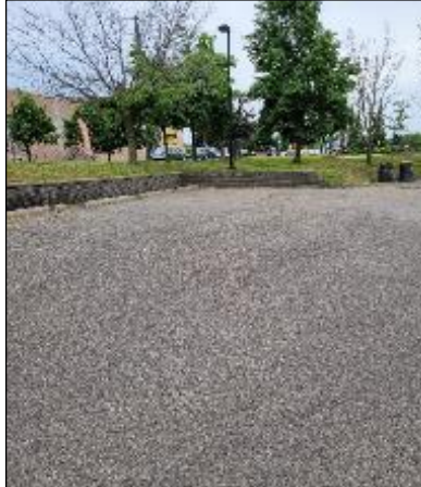
Photo C17: Southeast parking lot looking southerly. Longitudinal cracking, alligator cracking, eroding asphalt, retaining wall in background.
