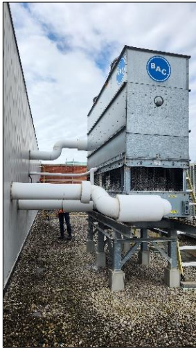
Photo M7: Cooling Tower
