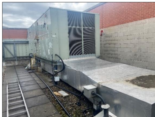
Photo M14: RTU-1 – Serving Gymnasium
