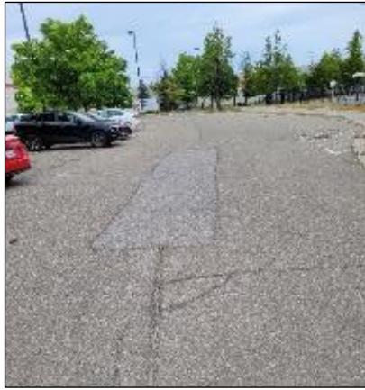
Photo C10: West Parking – Looking north from south end, cracking, previously sealed, patching, asphalt erosion. CB7 top right.
