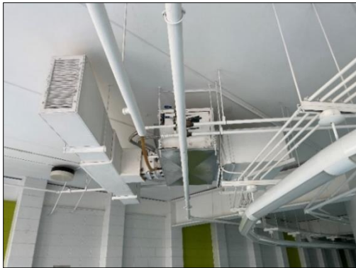
Photo M13: Typical Water Source Heat Pump
