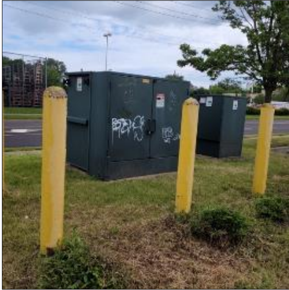
Photo E1: Hydro Transformer
