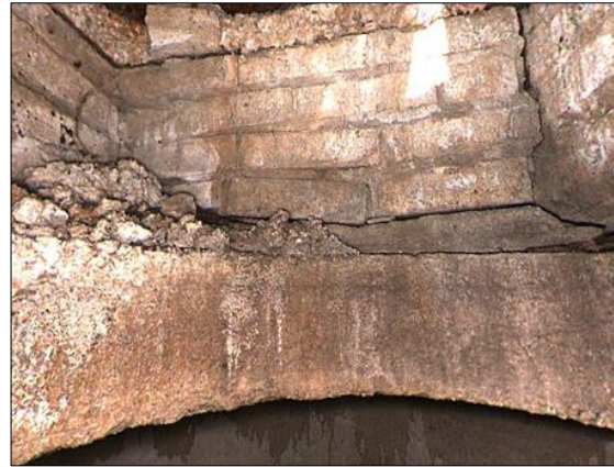
Photo C61: SAN MH2: Cracked adjustment rings mortar bed.
