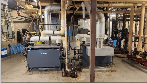
Photo M6: Steam Boilers Serving Steam Rooms
