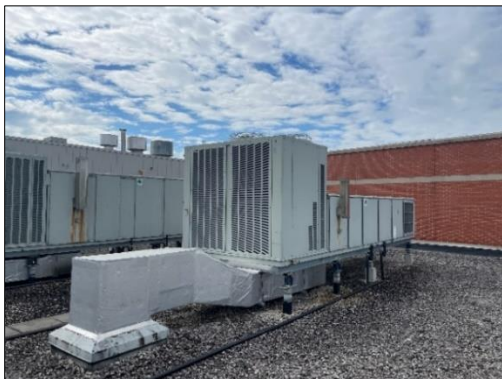
Photo M15: RTU-2 and RTU-3 – Providing Ventilation for Change Rooms
