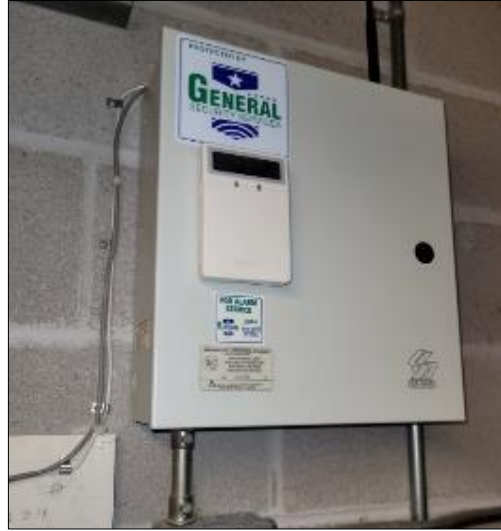
Photo E16: Main Security Panel
