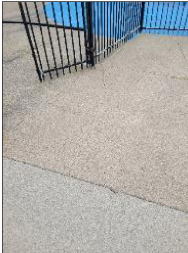
Photo C27: West at Splash Pad Entrance cracked sidewalk.
