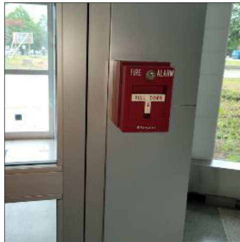
Photo E22: Typical Fire Alarm Pull Station at Exit Door
