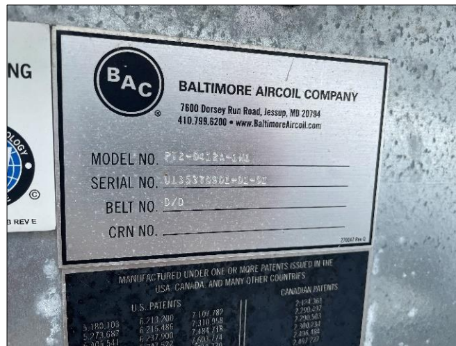
Photo M8: Cooling Tower Nameplate
