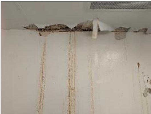
Photo ST 3: Leaking in laundry room.
