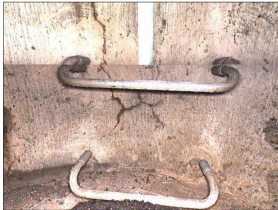
Photo C55: STMH 1: Cracks in MH
