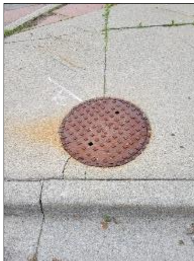
Photo C22: East Entrance – Sidewalk crack at SAN MH2. MH2 requires replacement of adjustment rings.
