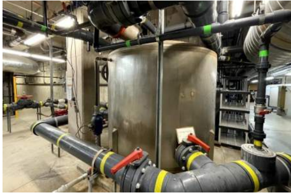
Figure 1 – Main Pool Balance Tank
