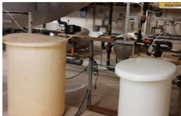
Figure 12 – Chlorine Storage Tanks
