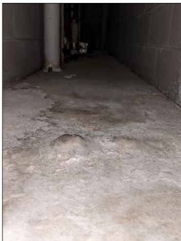
Photo ST 1: Slab on Grade Heaving
