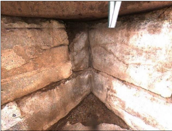
Photo C56: STMH 2: Cracks Riser/Adjustment Ring
