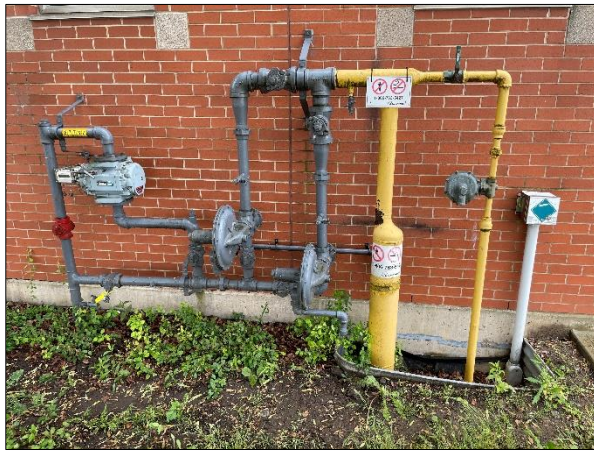
Photo M1: 2 PSI incoming gas service meter and regulator.
