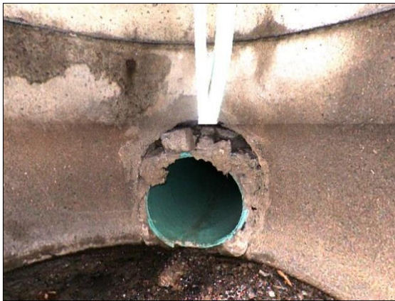
Photo C48: CB 2: Joint Seal
