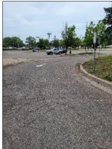
Photo C20: East Entrance – Extensive cracking & asphalt erosion, loss of asphalt
