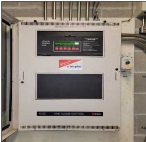
Photo E19: Main Fire Alarm Control Panel
