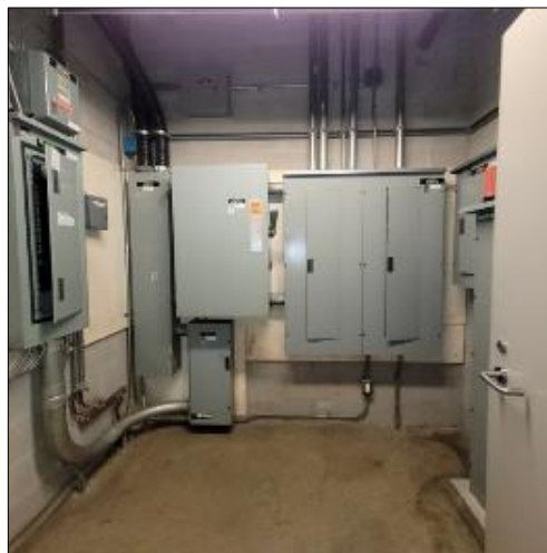
Photo E4: Typical Distribution Equipment in Elec Rooms
