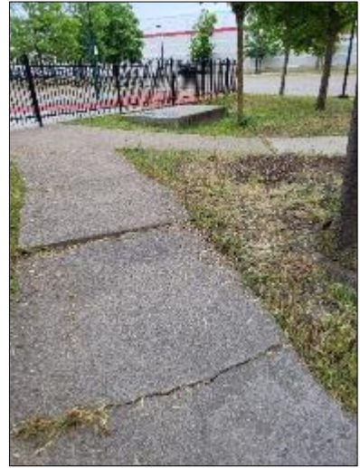
Photo C26: Northeast Entrance to Splash Pad: Sidewalk heaved and broken, differential settlement.
