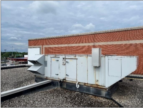
Photo M19: RTU-7 - Serving 2 nd Floor Addition
