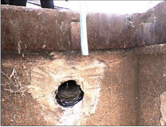
Photo C52: CB 8: Damage to CB structure, mortar bed failure.
