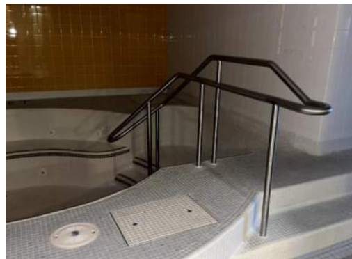
Figure 38 – Typical Whirlpool Handrails
