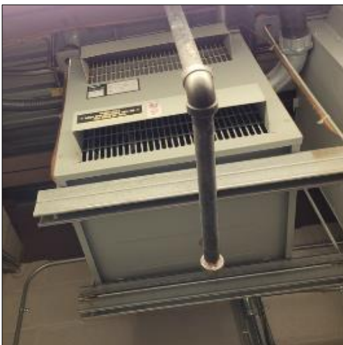
Photo E3: Typical Ceiling Mounted Transformer in Elec Rooms
