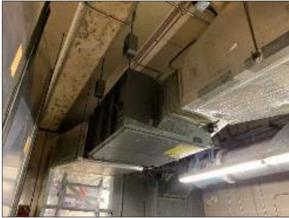
Photo M22: AHU-2 Serving ventilation for laundry room.
