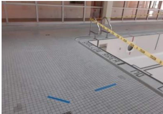
Figure 20 – Main Pool Deck, Marked Location of Severe Delamination
