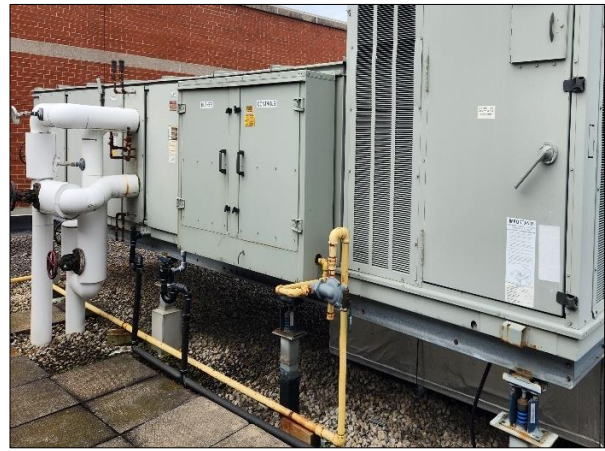
Photo M2: Typical gas piping connection to equipment with regulator.
