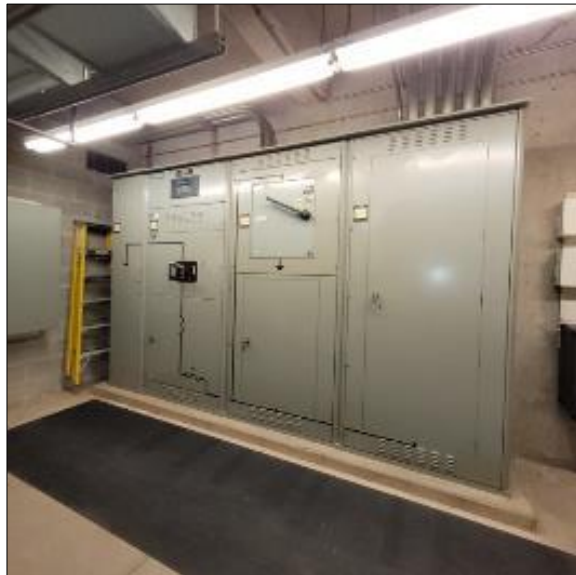
Photo E2: Main Switchboard
