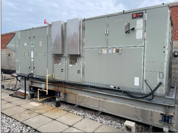
Photo M17: RTU-5 – Serving Second Floor Fitness and Upper Main Lobby
