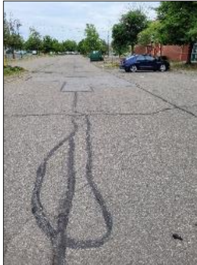
Photo C8: North Parking looking east from area of transformer. STMH 3 and CB5 in background. Longitudinal cracking, some previously sealed and sealing failing, patching at MH and CB.
