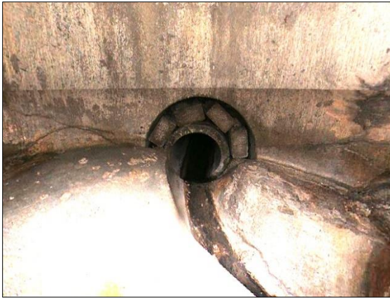
Photo C60: STMH 5: Structure Cracks
