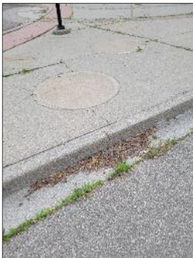
Photo C21: East Entrance – Sidewalk cracked, differential settlement sidewalk, curb.
