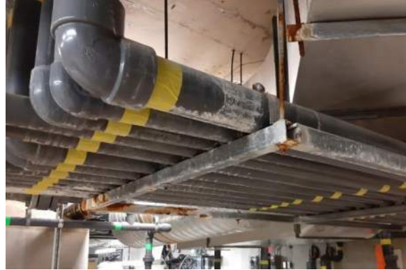
Figure 14 – Corroded Pipe Supports
