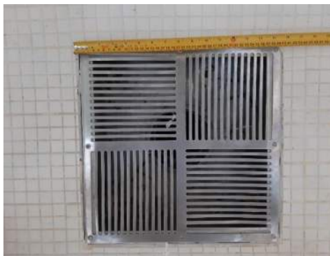
Figure 26 – Main Pool Main Drains
