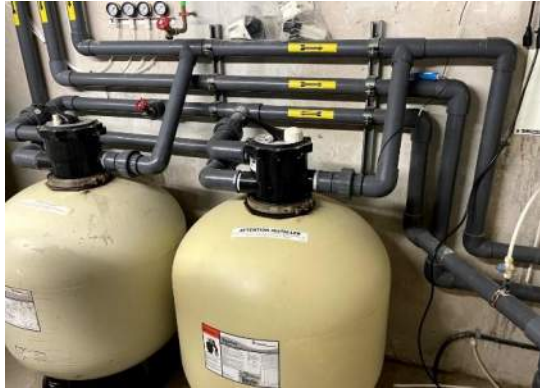
Figure 9 – Splash Pad Vertical Sand Filters
