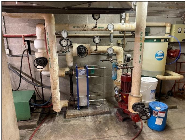
Photo M24: Glycol Heat Exchanger, Pump and Feed Tank Serving AHU-1.
