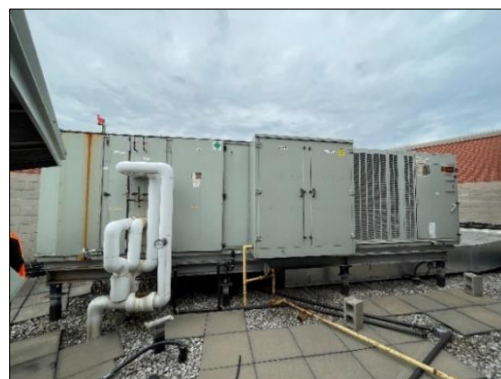
Photo M16: RTU-4 – Serving Ventilation Air for Water Source Heat Pump Units
