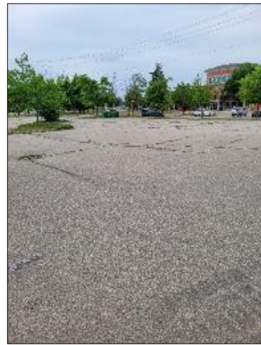
Photo C3: East parking lot looking from northeast corner of property southwesterly. Cracking, grass growing in cracks. Oxidized asphalt. CB1 mid picture, at left.
