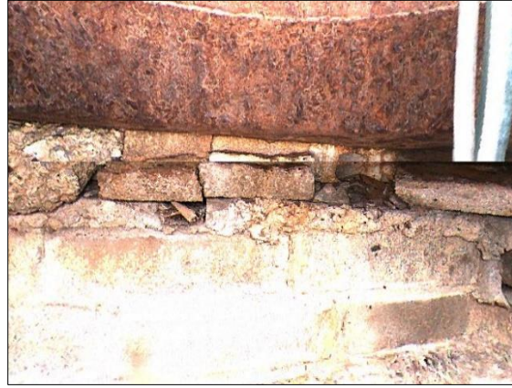
Photo C59: STMH 5: Mortar bed/adjustment ring cracked.
