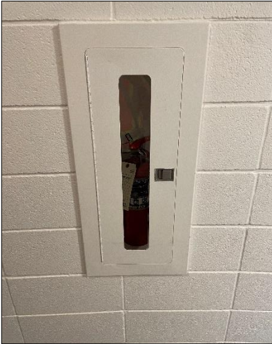
Photo M27: Typical Recessed Fire Extinguisher Cabinet
