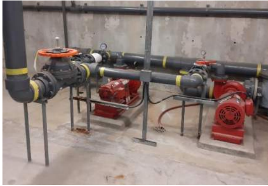
Figure 3 – Main Pool Filter Pumps
