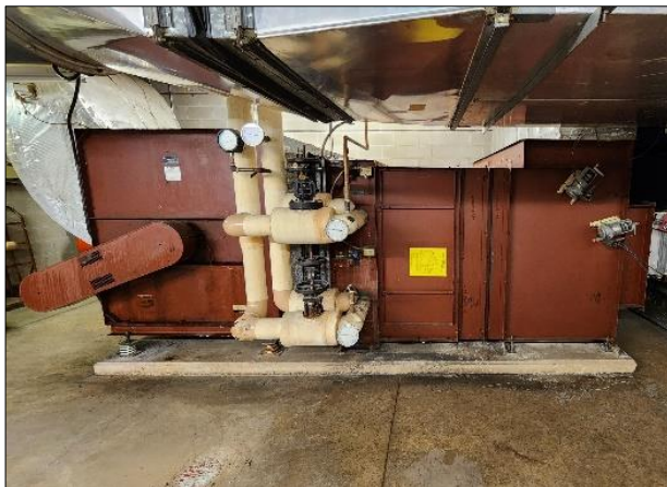
Photo M20: AHU-1 Swimming Pool Unit
