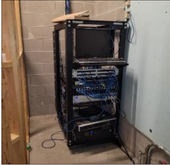
Photo E15: Main IT Rack in Elevator Machine Room
