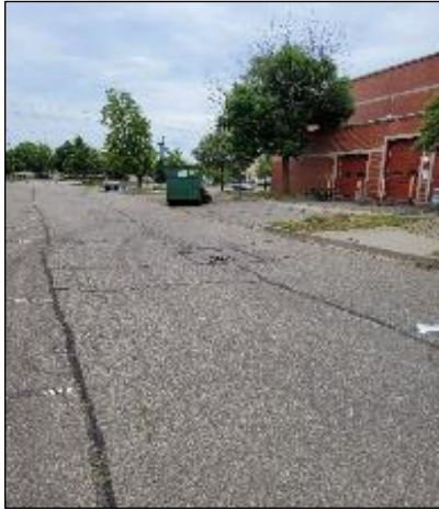
Photo C4: North Parking lot looking east near north entrance. Alligator cracking along longitudinal cracks, longitudinal cracking 5.5 m off curb, patching CB 5.
