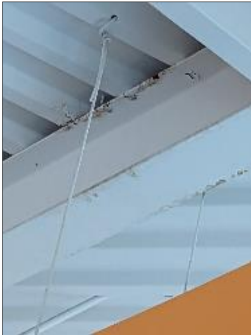
Photo ST 7: Signs of water damage on structural framing.
