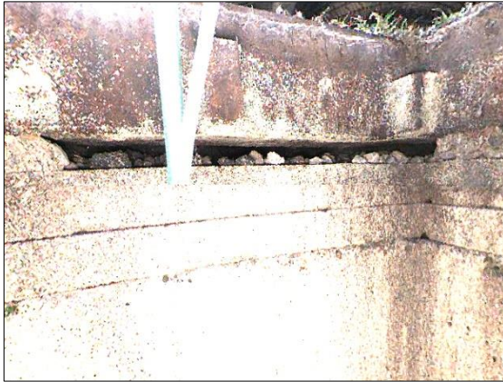
Photo C46: CB 1: Frame mortar bed failure, typical of bed failures. Adjustment rings.
