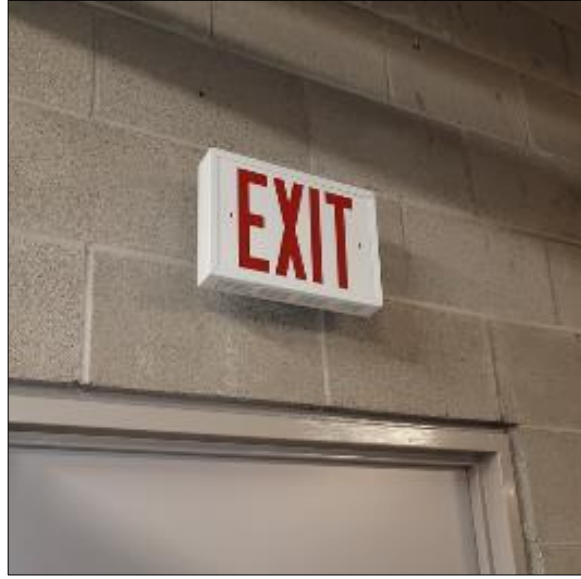
Photo E14: Typical Exit Sign
