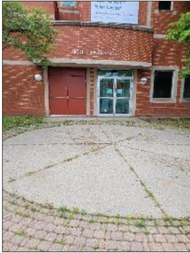
Photo C24: North Entrance –Sidewalk and interlocking block settled relative to each other.
