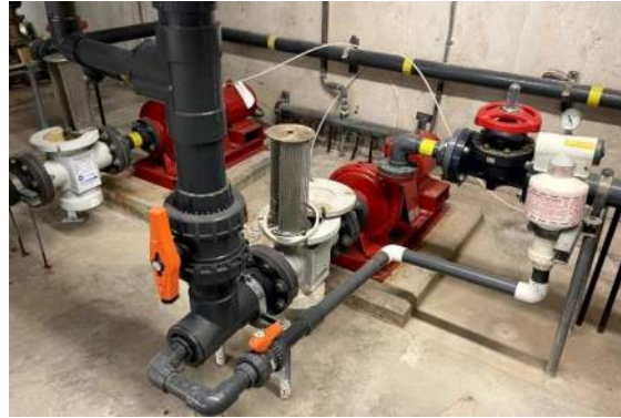
Figure 4 – Whirlpools’ Filter Pumps
