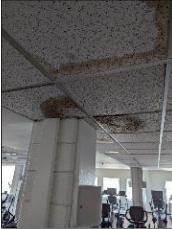
Photo ST 5: Leaking through ceiling tile.
