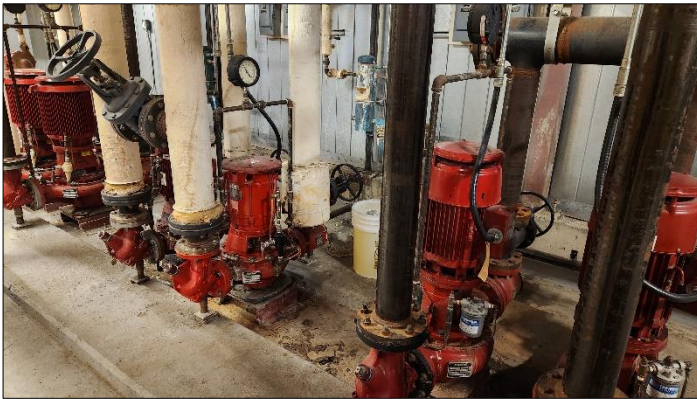
Photo M9: Pumps P-5, P-6, P-7, P-8, P-9 and P-10
