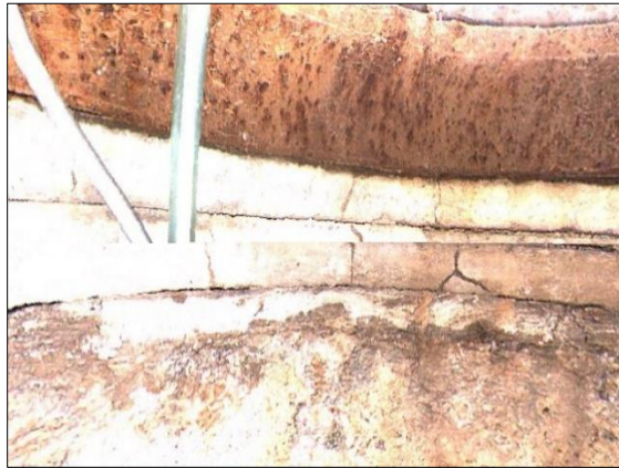
Photo C57: STMH 3: Adjustment Ring Cracks
