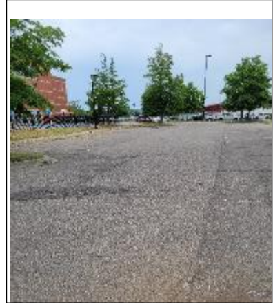
Photo C12: West Parking – North end, looking south, alligator and longitudinal cracks with grass growing.
