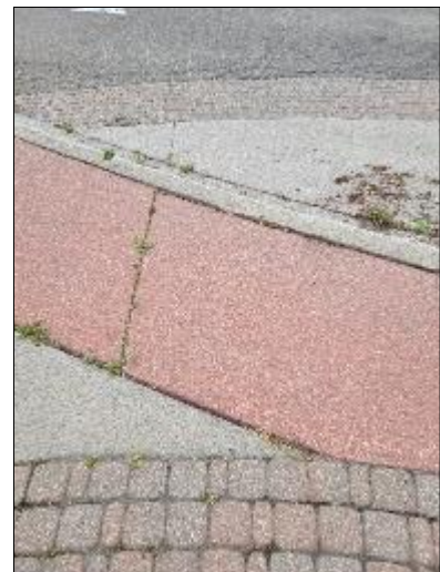
Photo C23: East Entrance – Sidewalk cracked, concrete and interlocking brick settled relative to each other and curb.
