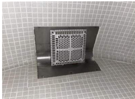
Figure 27 – Typical Whirlpool Main Drain
