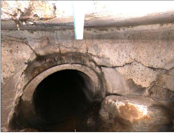
Photo C58: STMH 3: Structure Cracks
