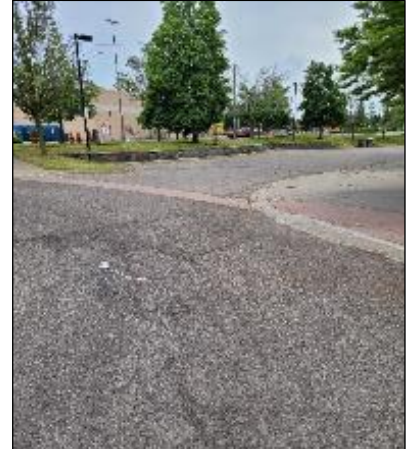
Photo C18: East Entrance – Extensive cracking & asphalt erosion.
