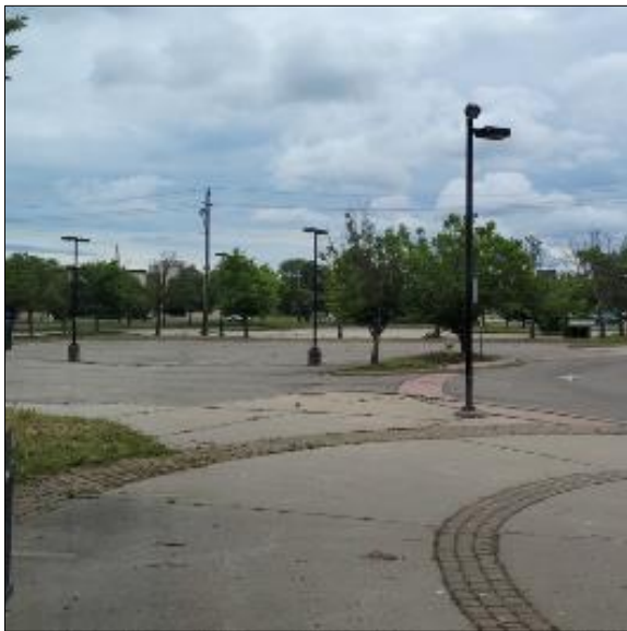
Photo E11: Typical Exterior Lighting Fixtures on Pole
