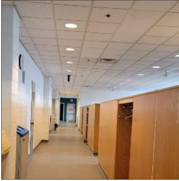
Photo E9: Typical Lighting Fixtures in Gym and Change Rooms
