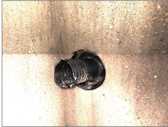
Photo C47: CB 1: 100 mm HDPE weeper with joint seal.
