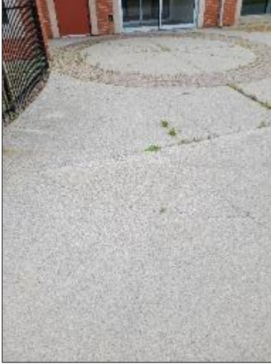
Photo C30: South Entrance – Cracked sidewalk, differential settlement.
