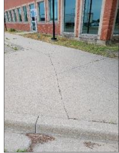
Photo C32: Southeast Corner – Cracked sidewalk, differential settlement.
