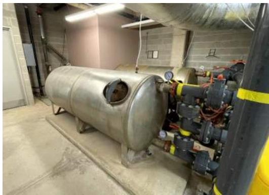
Figure 7 – Main Pool Horizontal Sand Filters
