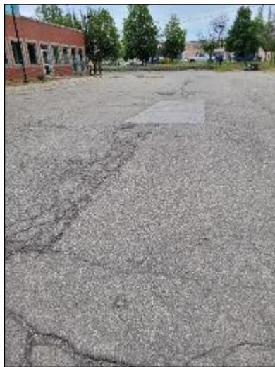
Photo C13: South Parking Lot Looking East to CB8 – Extensive cracking, patching, asphalt erosion, asphalt loss.
