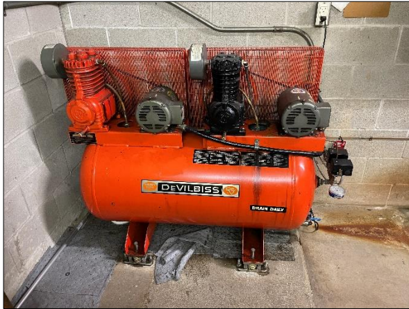
Photo M25: Pneumatic Controls Air Compressor
