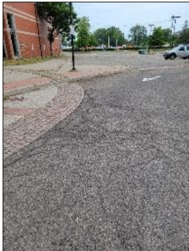
Photo C19: East Entrance – Extensive cracking & asphalt erosion
