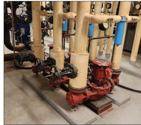
Photo M10: Pumps P-1 and P-2
