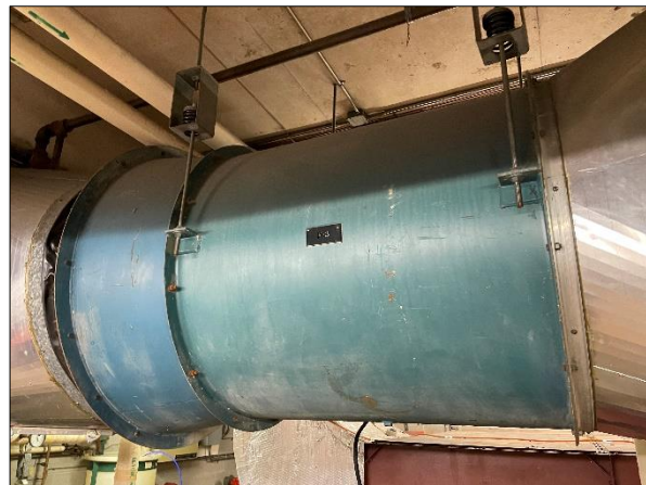
Photo M21: F-3 Swimming Pool Exhaust Fan
