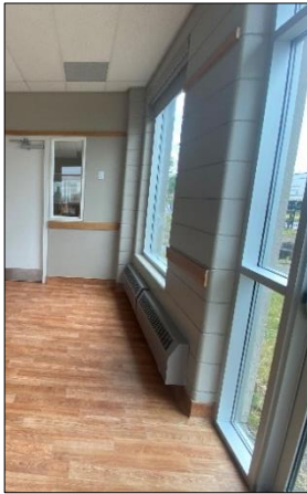
Photo M11: Typical Wall Finned Baseboard Heater
