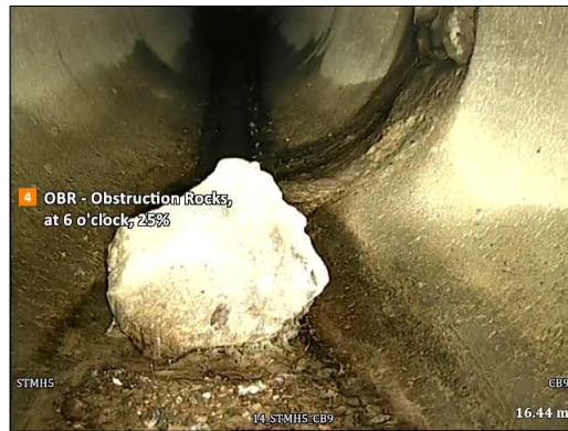
Photo C45: STMH 5 – CB 9: Debris in pipe, lead from CB 8 top right.
