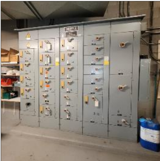
Photo E5: MCC 1 in 3 rd Floor Mechanical Room
