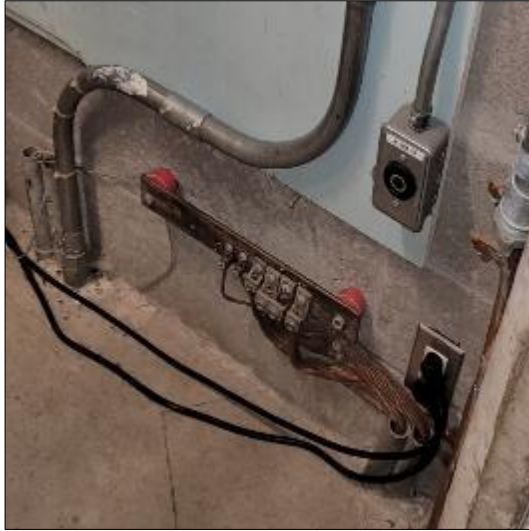
Photo E23: Grounding Busbar in Elevator Machine Room
