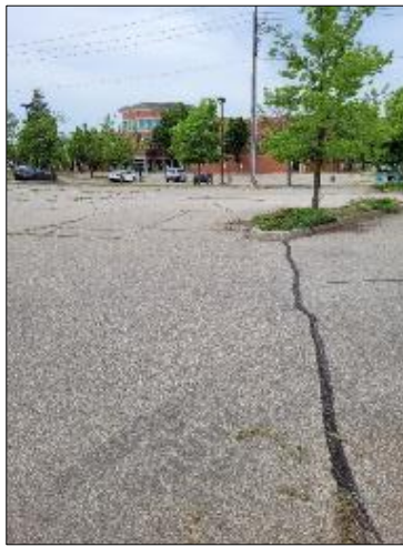
Photo C2: East parking lot looking from northeast corner of property southwesterly. Cracking, grass growing in cracks. Oxidized asphalt. CB1 in mid picture.
