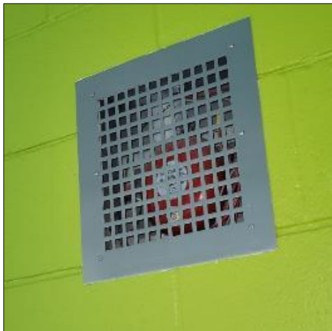
Photo E21: Typical Fire Alarm Bell in Common Area
