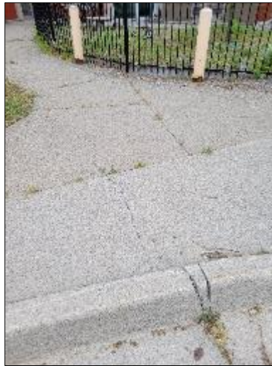
Photo C28: West Entrance – Cracked sidewalk and broken curb. Sidewalk settled relative to curb.
