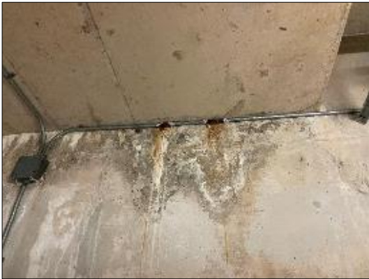
Photo ST 4: Signs of leaking through Slab.
