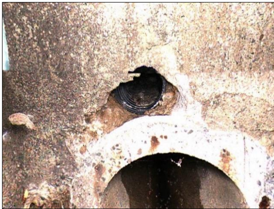
Photo C49: CB 3: Weeper connection above storm pipe.
