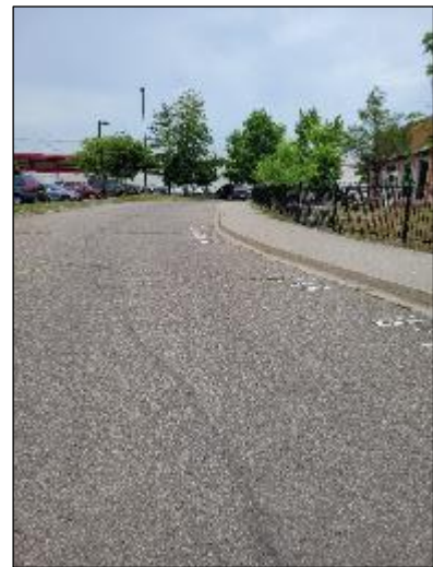
Photo C15: South Entrance Looking West – Better condition than to east. cracking, cracks sealed and sealing failing, asphalt erosion.
