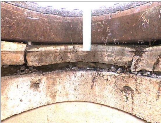
Photo C54: STMH 1: Adjustment ring crack and mortar bed failure.
