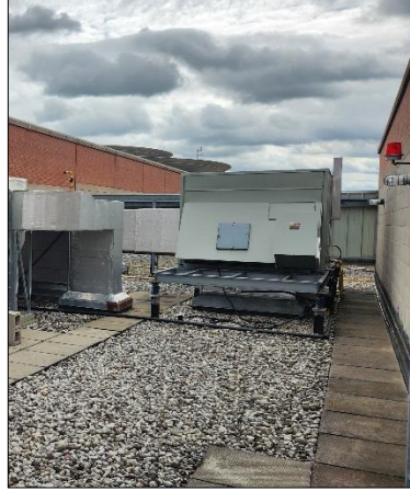
Photo M18: RTU-6 – Serving Ground Floor Lobby
