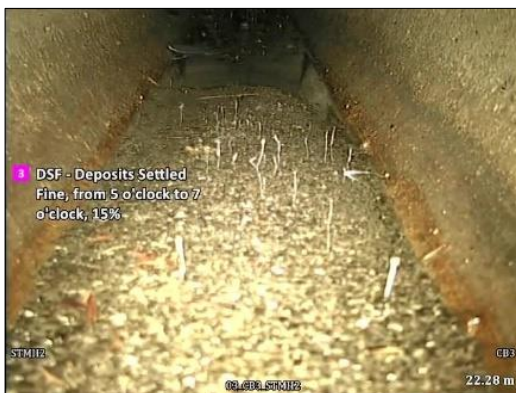
Photo C40: Lead CB 3 to STMH 2: Deposits in pipe.
