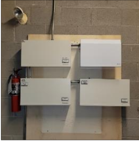
Photo E13: Typical Remote Heads and Battery Units
