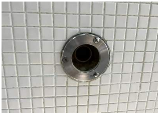
Figure 30 – Main Pool Return Fitting, Missing Eyeball
