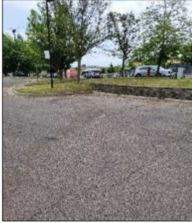
Photo C16: Southeast parking lot looking northeasterly. Longitudinal cracking, eroding asphalt, retaining wall in background.
