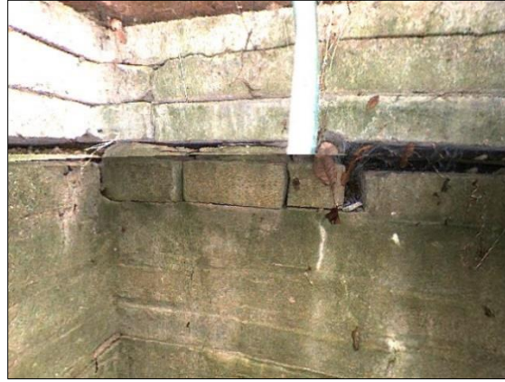
Photo C53: CB 10: Cracked adjustment units/riser.
