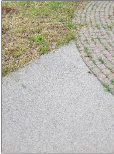
Photo C25: North Entrance – Bolts sticking up in sidewalk.
