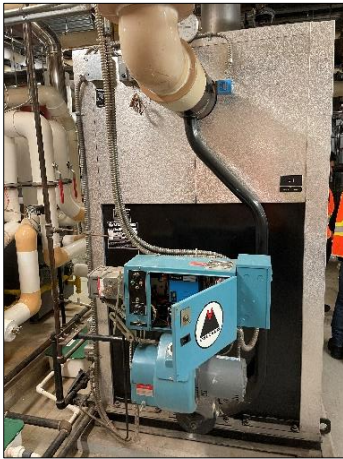
Photo M3: Boiler #1
