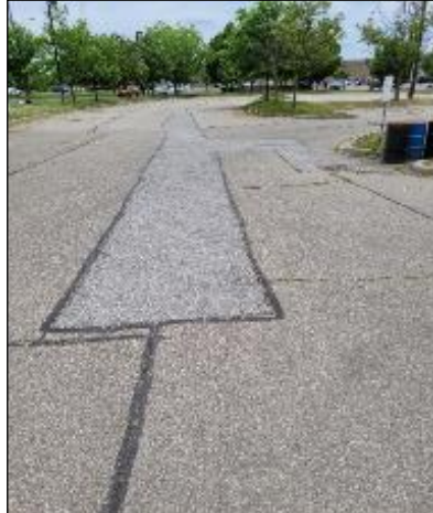
Photo C5: North Parking Lot looking east from northeast entrance. CB 4 in background, patching down center of lot and around CB, longitudinal cracks, some sealed. Grass in others.
