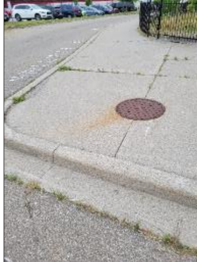
Photo C31: South Entrance – Cracked sidewalk. STMH 5 requires replacement of adjustment rings, differential settlement.
