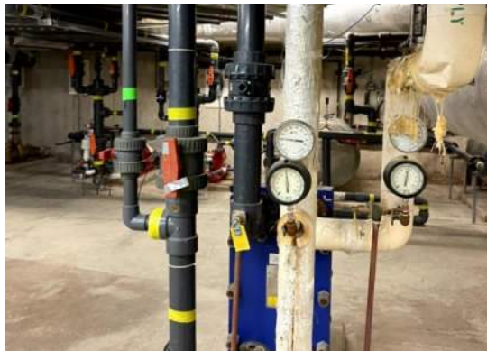
Figure 16 – Main Pool Heat Exchanger
