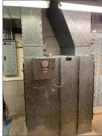
Photo M23: Laundry Dryer Lint Filter Unit
