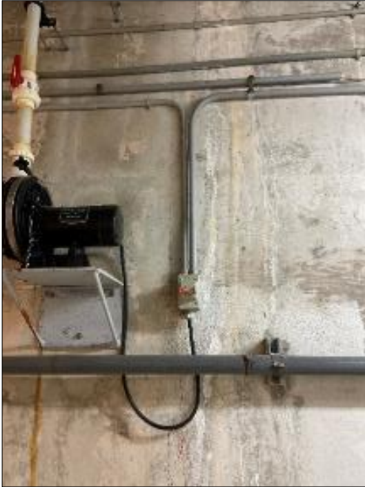
Photo ST 2: Signs of leaking through pool wall.
