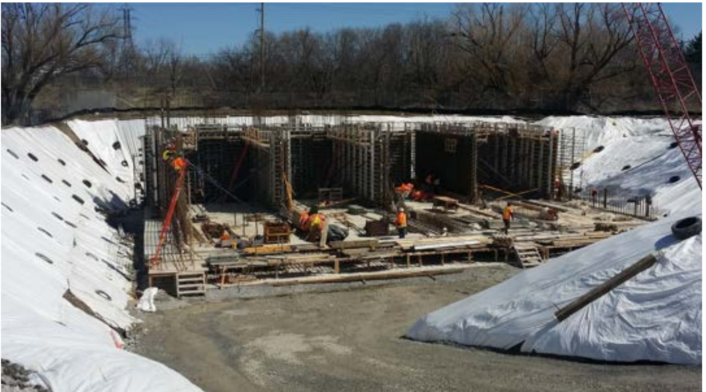
Figure 5: Glengarry Road CSO Tank
