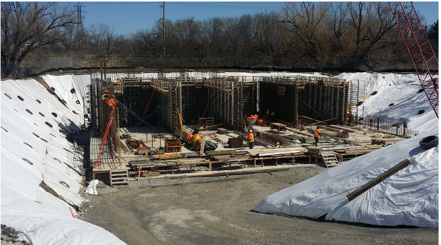
Figure 5: Glengarry Road CSO Tank
