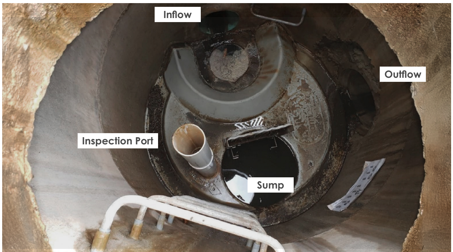
View looking down inside the manhole chamber into the OGS device.
