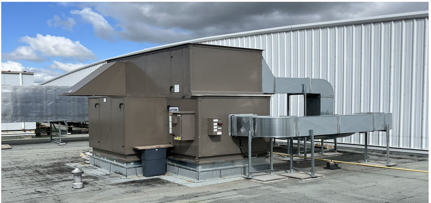
Seymour-Hannah Arena Dehumidification Units
