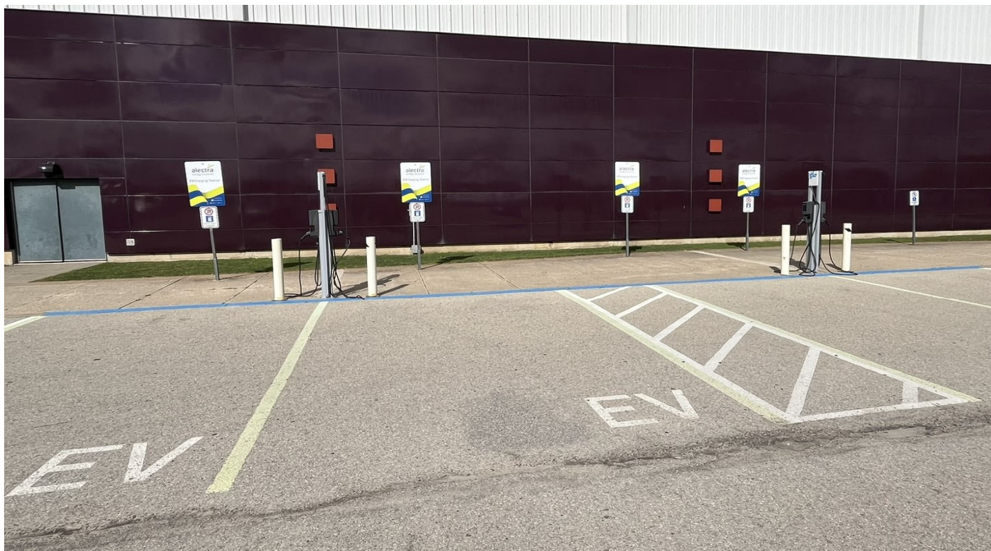
Newly Installed EV Charging Stations
