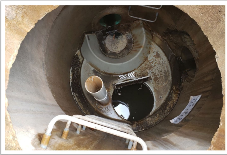
Figure 5: Typical OGS Configuration – View looking down inside the manhole chamber into the OGS device.
