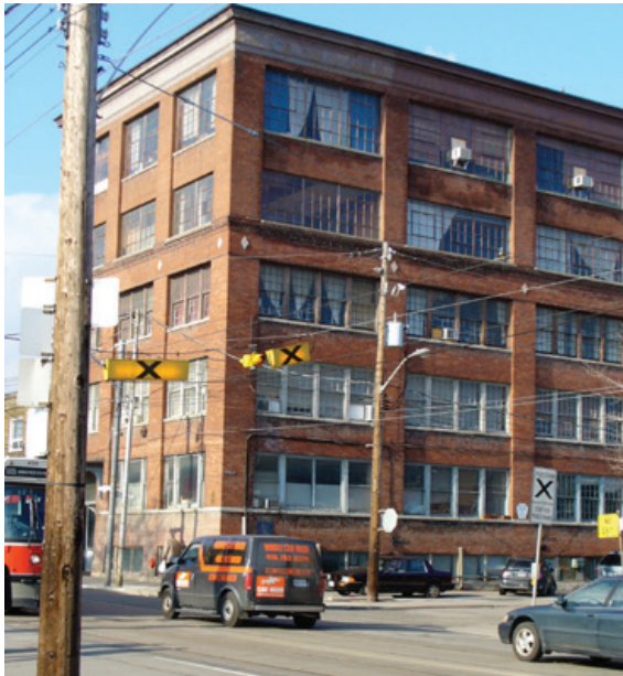
Toronto example of an Edwardian heavy masonry construction building that has had a two storey addition on the roof. (Catherine Nasmith)
