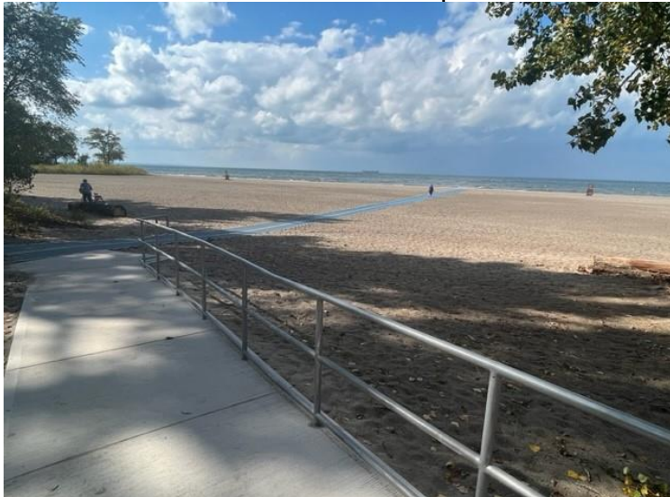
Mobi-Mats added on the beach to provide accessibility to the water's edge
